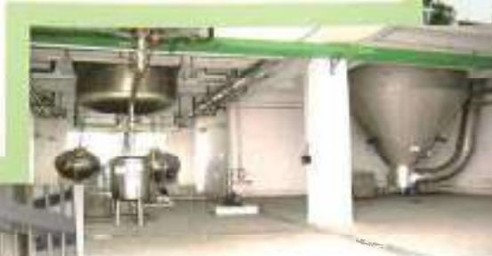
High Pressure Feed Pump to Spray Dryer
